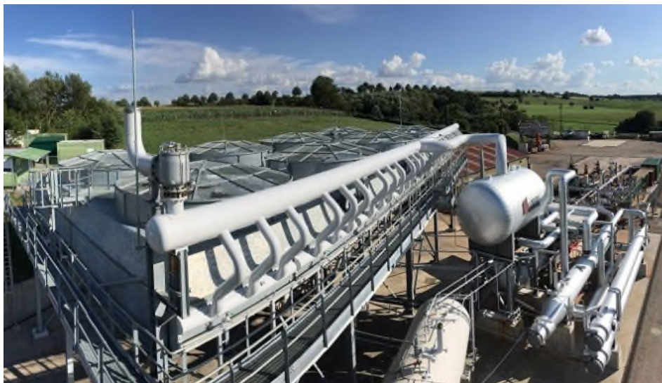
Figure 1: View of the Soultz-sous-Forêts geothermal power plant [source és].
