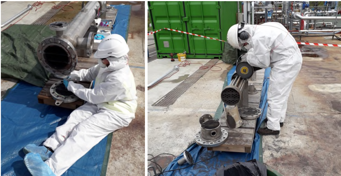
Figure 10: Prototype heat exchanger opening (left) and dismantling (right) [source és]
