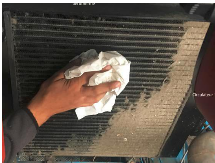
Figure 36: Cleaning operation of the air condenser
